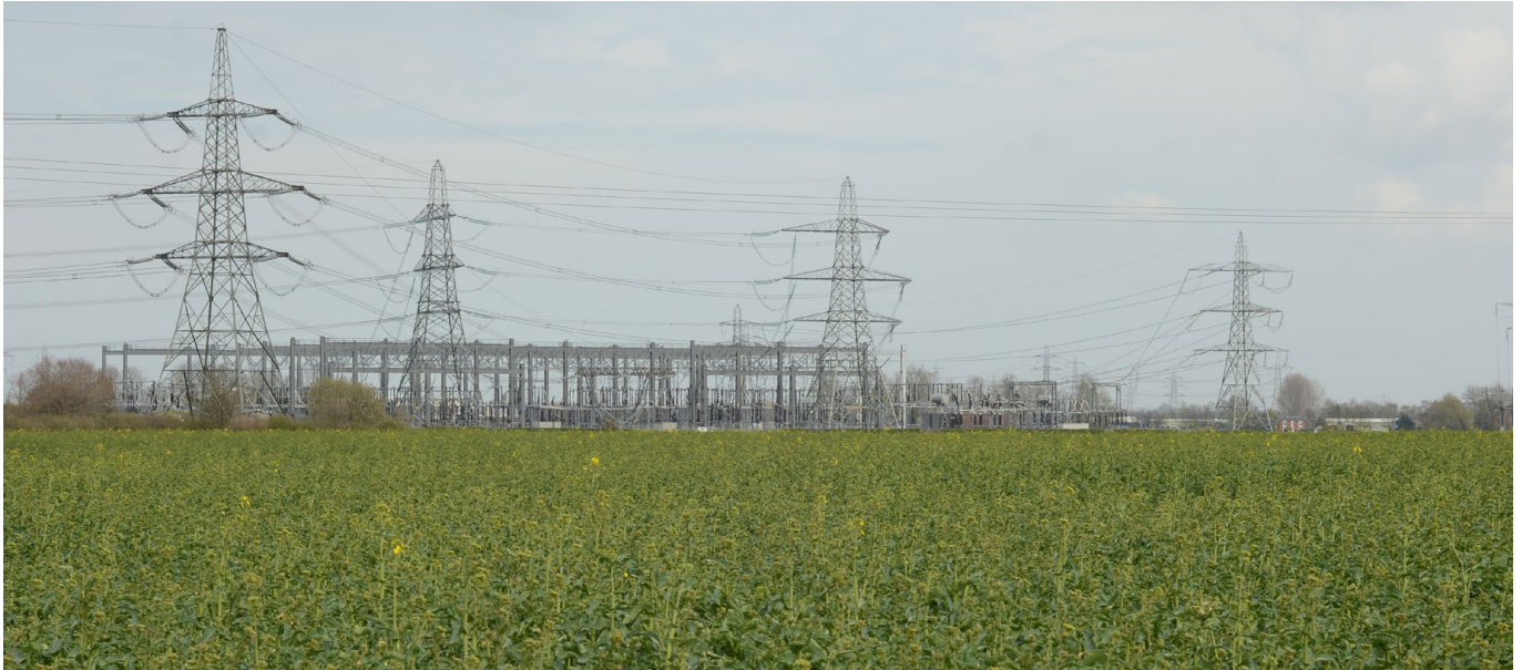
Img 3 - Creyke Beck Substation, approximately 180m east of the OnSS site (Source: Orsted)
